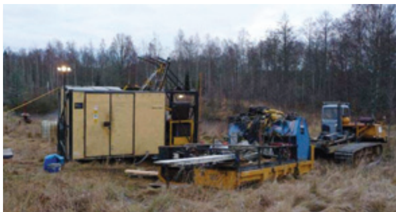
Tasman Crew Setting Up Drill Rig at Norra Kärr (Drilling commenced one month after company went public)
